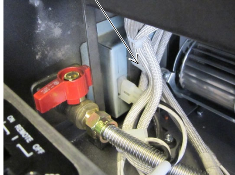
Junction Box (from inside fireplace)
