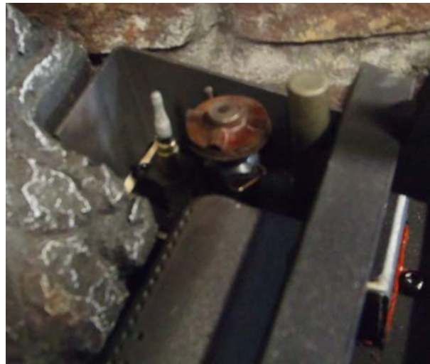
Figure 15. Pilot assembly beside the burner.
