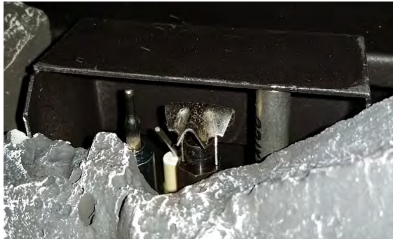
Figure 20: Pilot assembly beside the burner.
